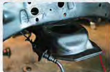
13 Moving to the front of our '65 Chevy, the first thing to do is remove all the factory components. We simply removed the tie rod ends and unbolted the upper and lower control arms to remove it all together. In order for there to be clearance for the upper coilover mounts, the factory spring perch needs to be slightly modified. Using a pneumatic punch, Tyler was able to remove the original brace and grind off the old studs. The new CPP upper CNC-bent and laser-cut spring pocket bracket has the appropriate-sized hole already cut in it and all the hardware mounting holes as well.
