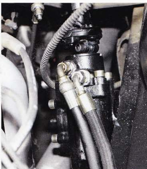
19. Power steering hoses are then attached to the new box, the system is bled, and in an afternoon, you've got 21st century steering under your classic Ford.
