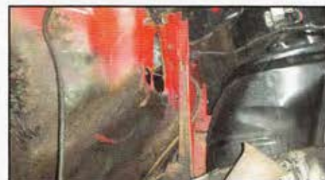
A view from the engine side looking at the firewall where the new column will be installed.
