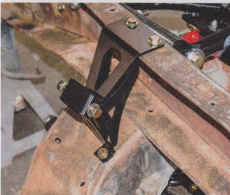
17 Made to bolt in place using existing holes from the old stock mounts, these beauties did just that with the supplied hardware.
